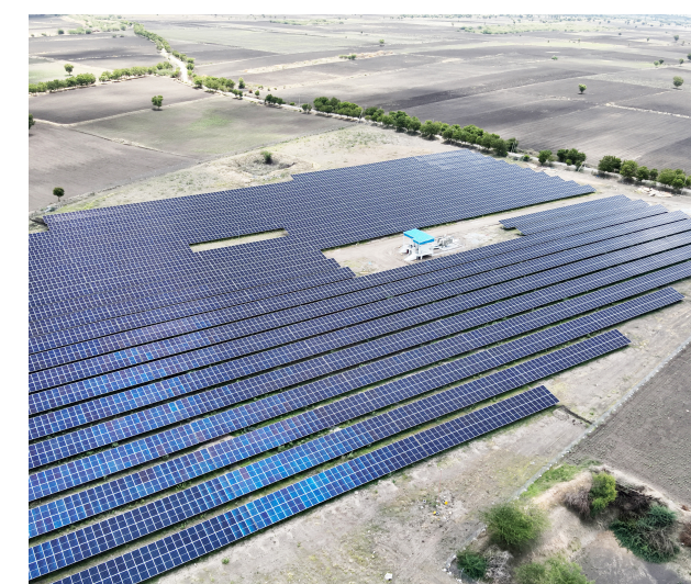
28 MWp Solar Project at Mundargi, Karnataka
