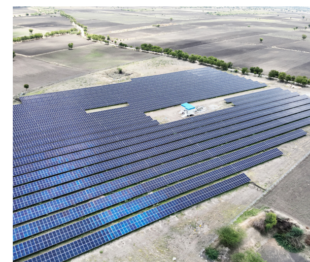
28 MWp Solar Project at Mundargi, Karnataka
